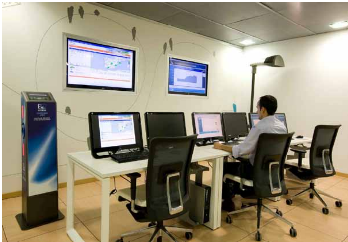
Smart Grid Service Center de Endesa
